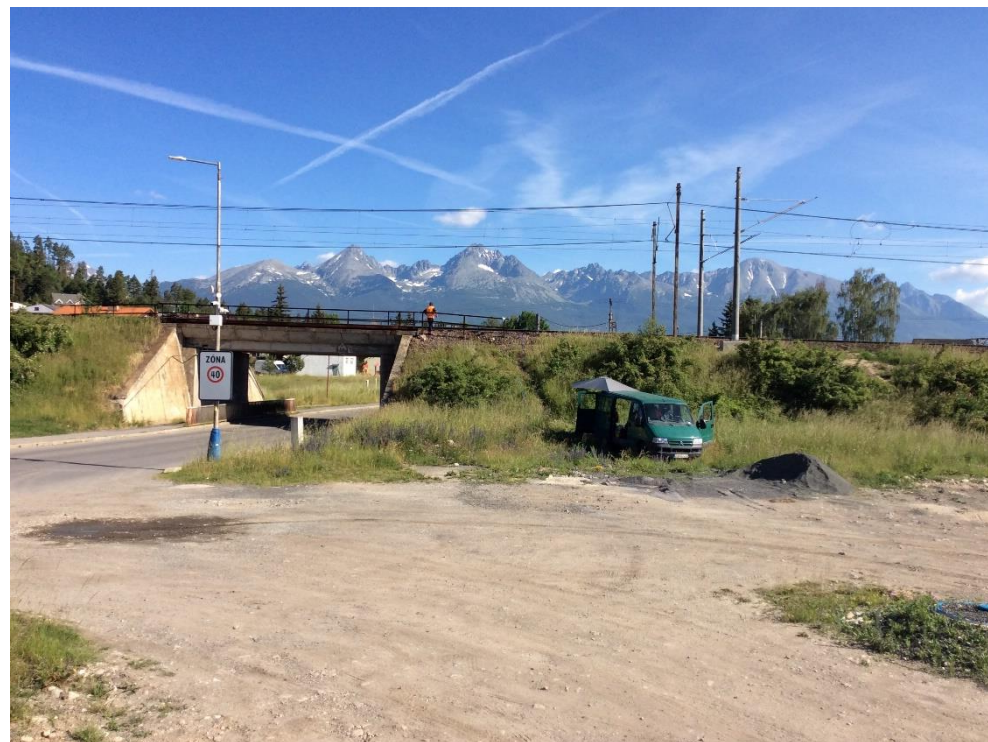
a) Monitoring of the transition zone of the bridge in front of the Svit station (state before modernization)
