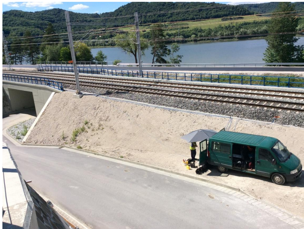
b) Monitoring of the transition zone of the bridge near the Miločov tunnel (state after modernization)
