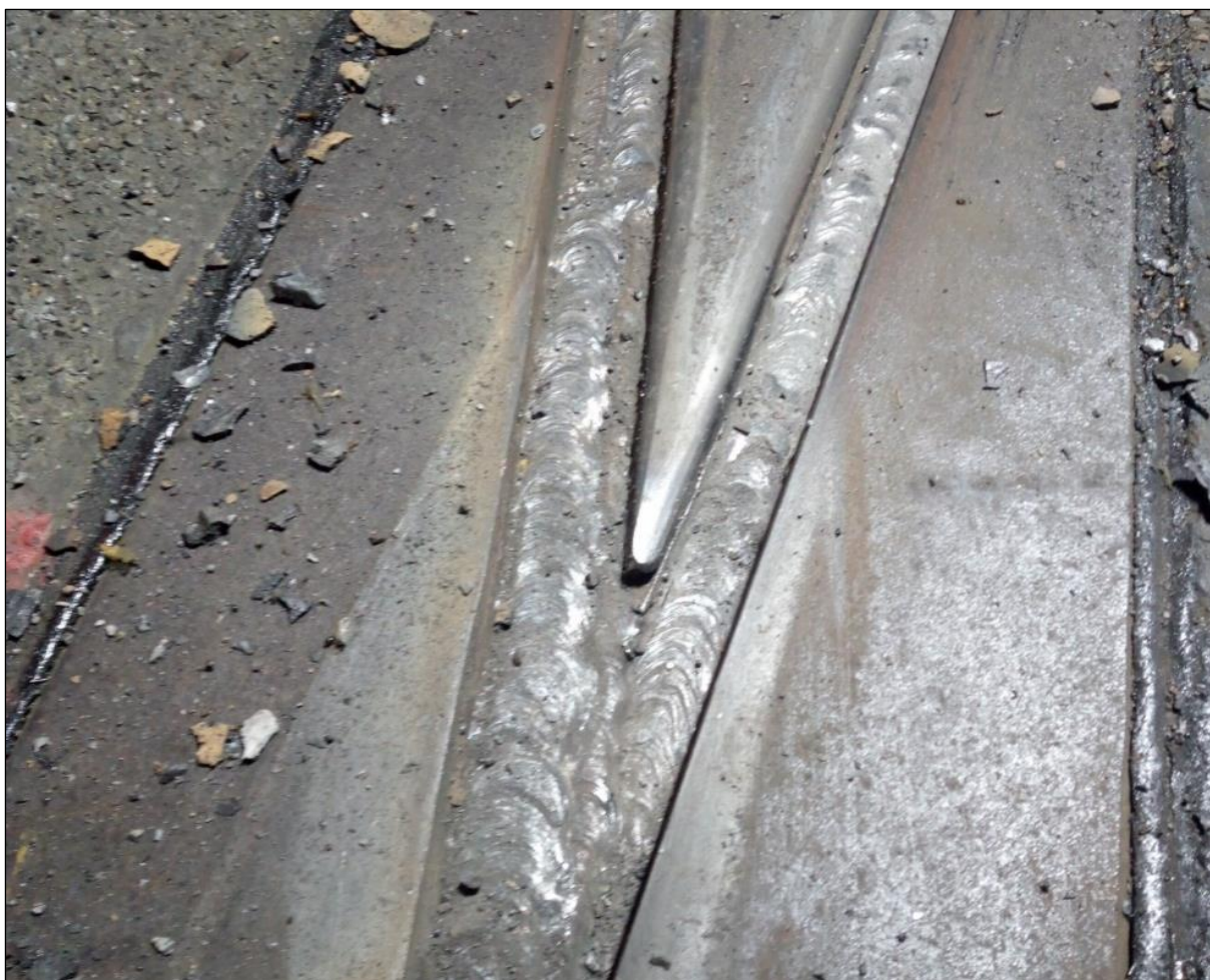
Fig.8 – Crossing Výtoň after welding and reprofiling. The transverse application of the caterpillars is noticeable
