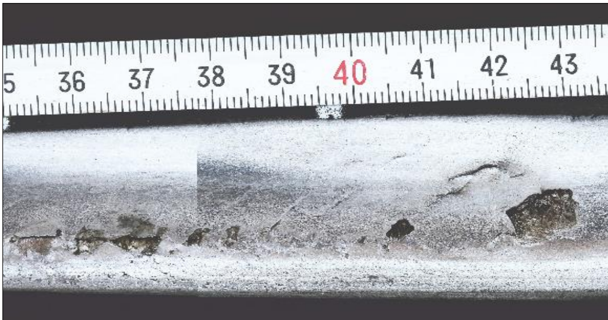
Fig. 1 – Sudden rail defect on the running surface of a switch frog (picture: [2])
